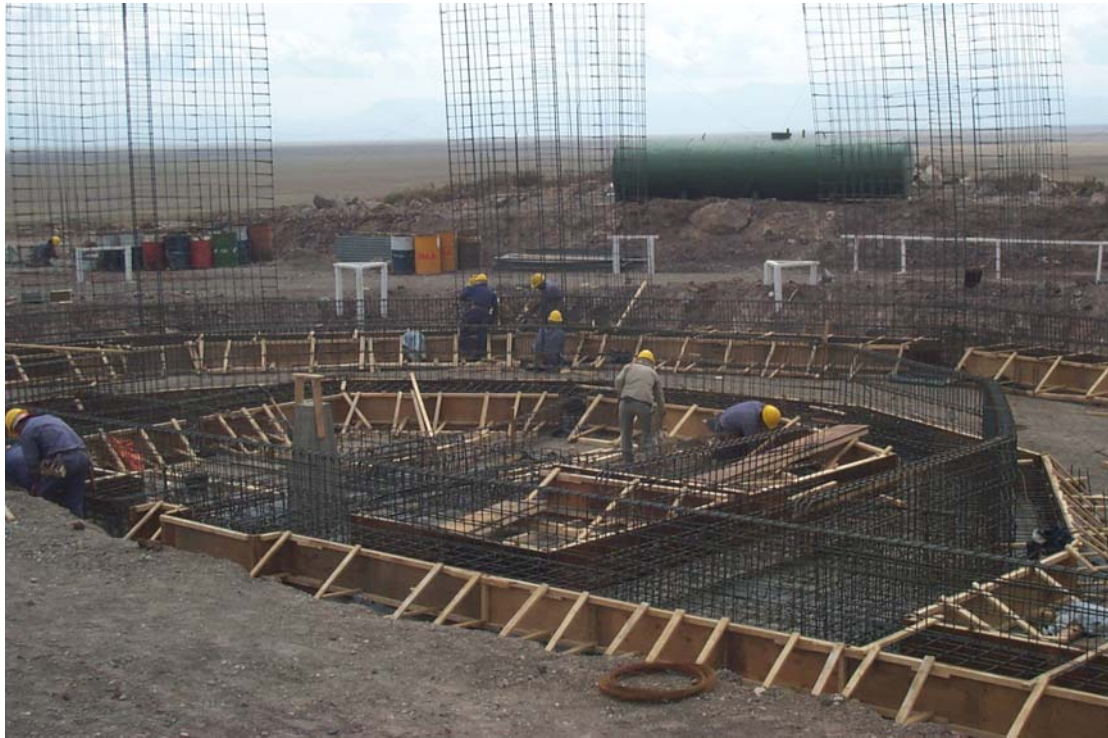
The monolith defines the reference point for the mirrors alignment
